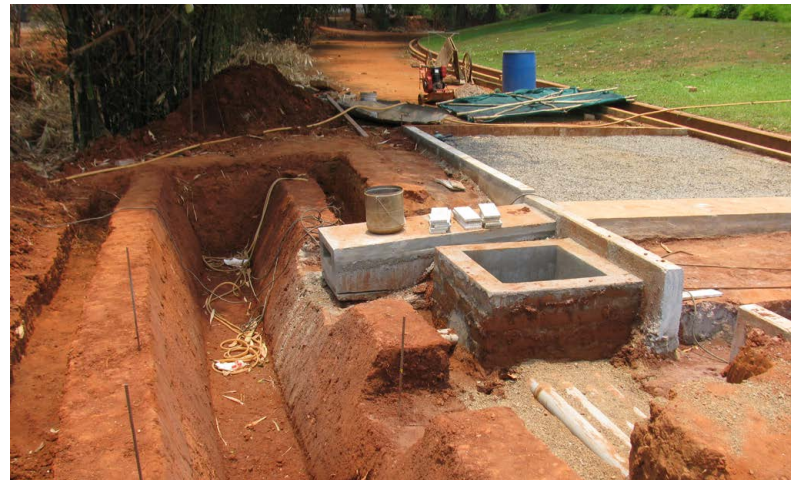
A trial sample of the open storm water collection channel being created at the edge of the oval road in April
