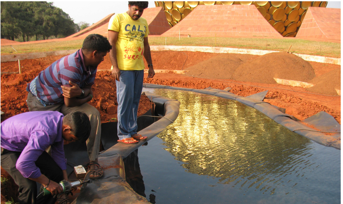
Work to install the HDPE pond liner on the elongated pond was carried out from Jan 17th to 19th.
