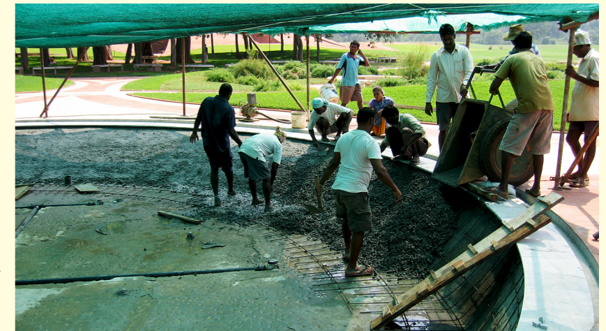
Final concreting in the pool in the Garden of Unity on November 12th
