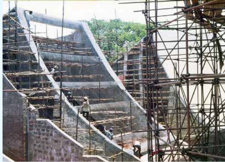
During the early 1990s the sweeping shapes of the 12 petals were constructed around Matrimandir as the labor force expanded to take up not only this work but also that of finishing the outer shells of Matrimandir.
