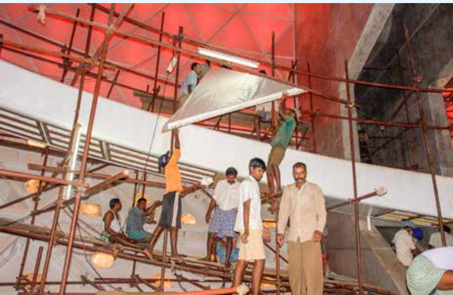
◀ Installation of the light-weight triangular panels of the interior skin took place in 2006-7.
