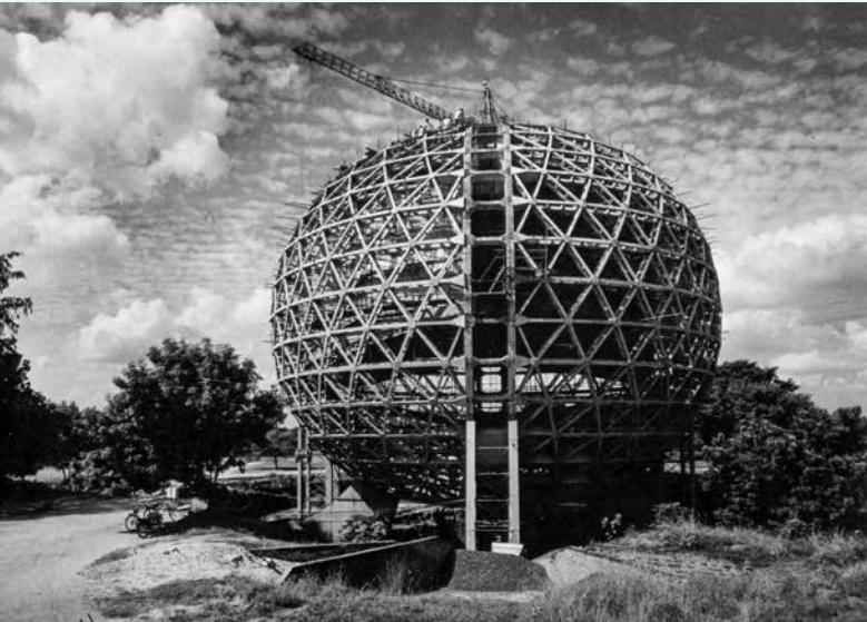
The spherical shell of the space frame was completed with the concreting of the top cap on 8th August 1988.
