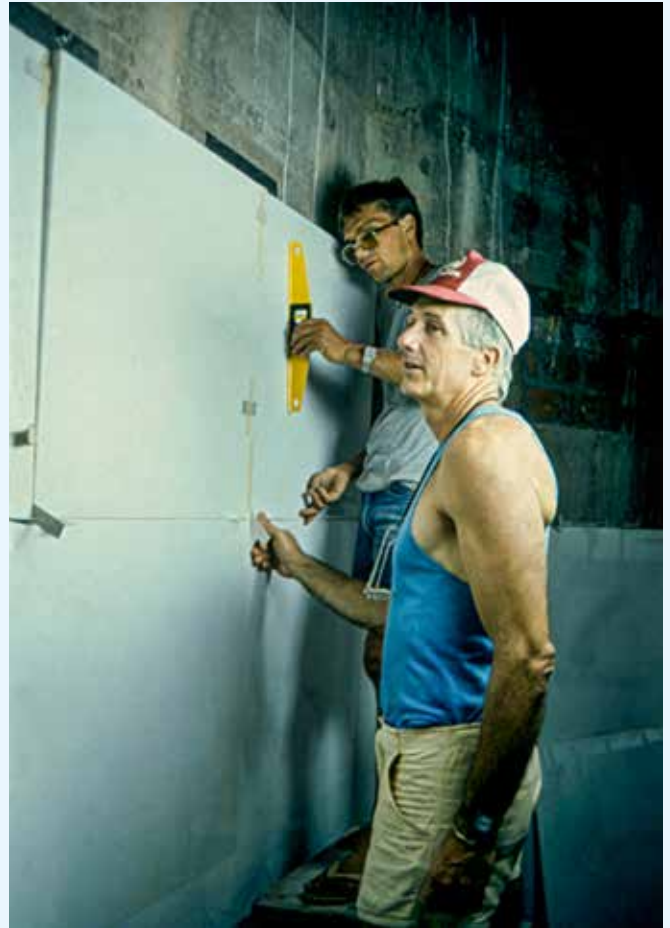
The polished white slabs of Italian marble were mounted on the Inner Chamber walls in 1989 - 90.
