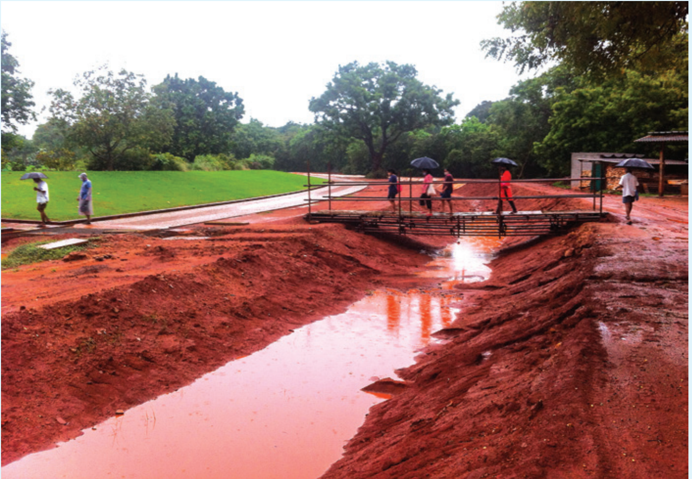
The rain water harvesting channel being built around the gardens is seen during a rainy day in July. Here it is still rough, unfinished: soon it will be waterproofed and given stone borders.
